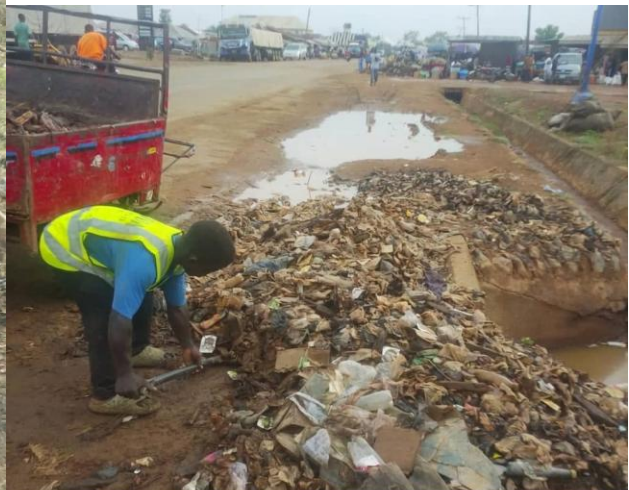
Evacuation of refuse from blocked drainage system by Ikom Urban Development Authority
