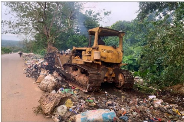
Evacuation of refuse by the roads side by Iikom Urban Development Authority
